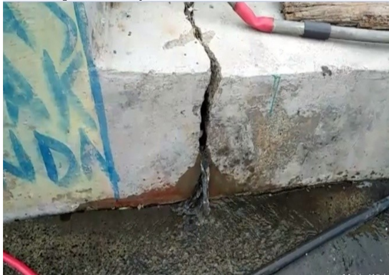
Figure 5. Crack in the water divider
